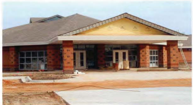
The school is a regular slab-on-grade building with concrete block walls and brick exterior.
